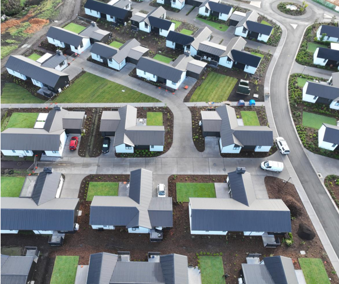
Te Puna Waioira, Kerikeri | Construction of the next stage of villas is progressing well to an expected FY23 delivery date. Planning is underway for an 800 sqm clubhouse with lounge, bar and activity amenity for residents' use.
