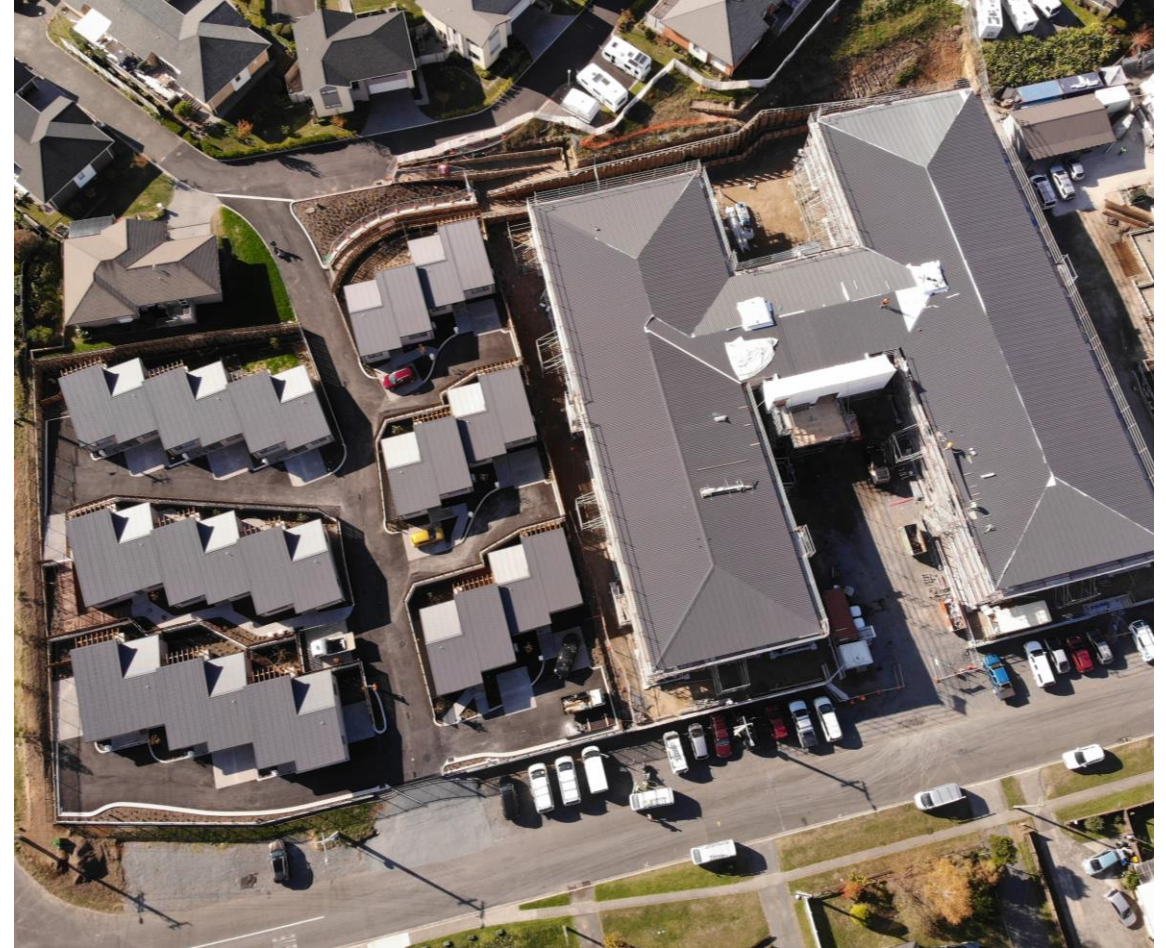
Lauriston Park, Cambridge | Construction of the care centre is progressing well. Roofing is advanced and internal fitout is progressing. 63 care suites will deliver up to hospital level care. The facility is programmed to complete in 4Q23.
