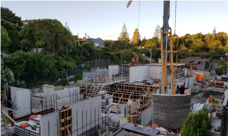
Aria Bay Apartments, Auckland
