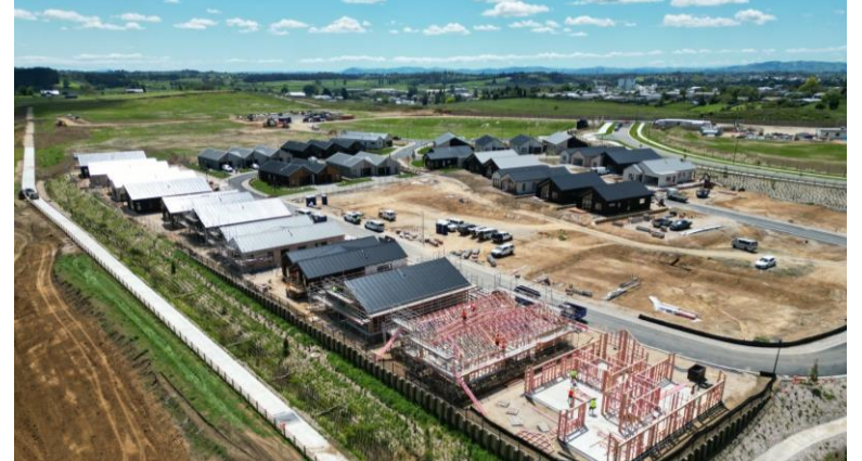
Whai Mauri Ora, Te Awamutu | villa construction Additional 16 villas to be delivered in 2H, site works continuing
