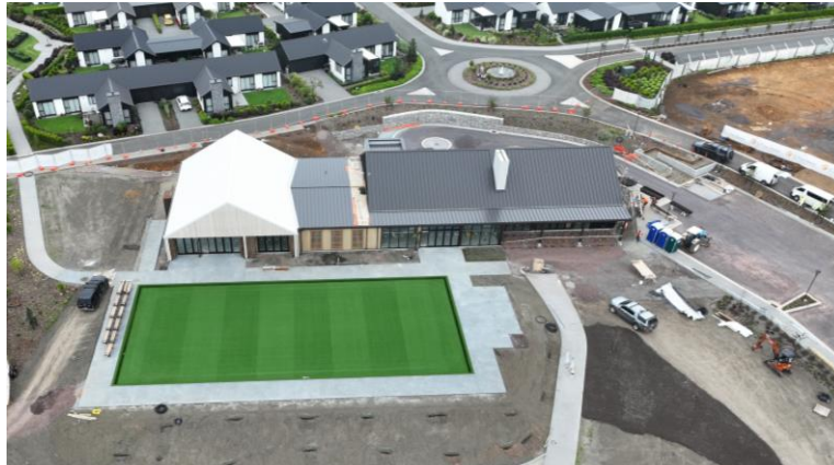
Te Puna Waiora, Kerikeri | Clubhouse Resident clubhouse due to complete in Jan 2024
