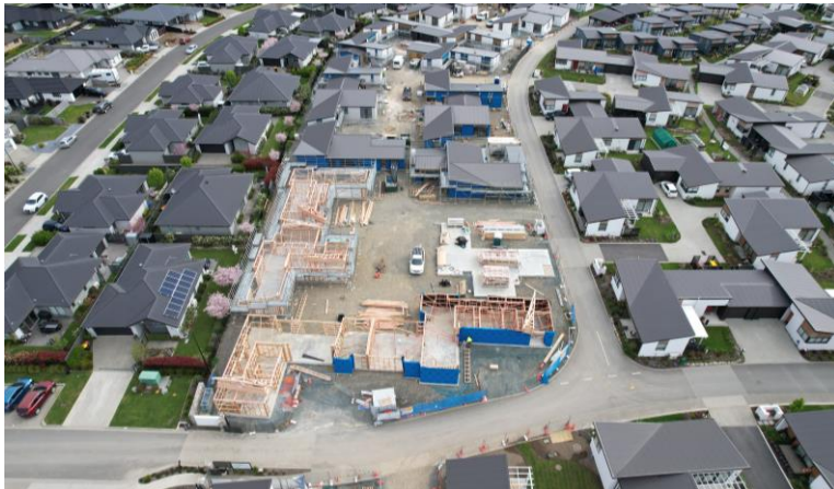
Waimea Plains, Richmond | villa construction On track to deliver 24 villas over 3Q and 4Q, ahead of programme
